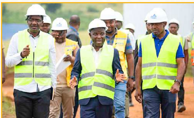
UDSM Vice Chancellor, Prof. William A. L. Anangisye (centre) when he visited UDSM-HEET buildings construction site in Kagera region. On his right side is Dr. Liberato Haule, UDSM-HEET Deputy Coordinator, and on his left is Eng. Benedict Chilla, Acting Director of Estate Services.
