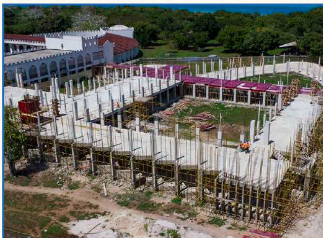
UDSM-HEET buildings construction site at the Institute of Marine Sciences (IMS), Buyu, Zanzibar.
